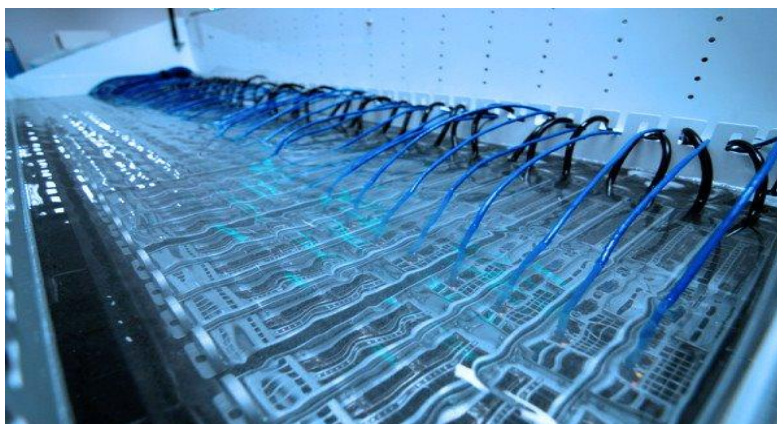
DATA Centre Cooling
